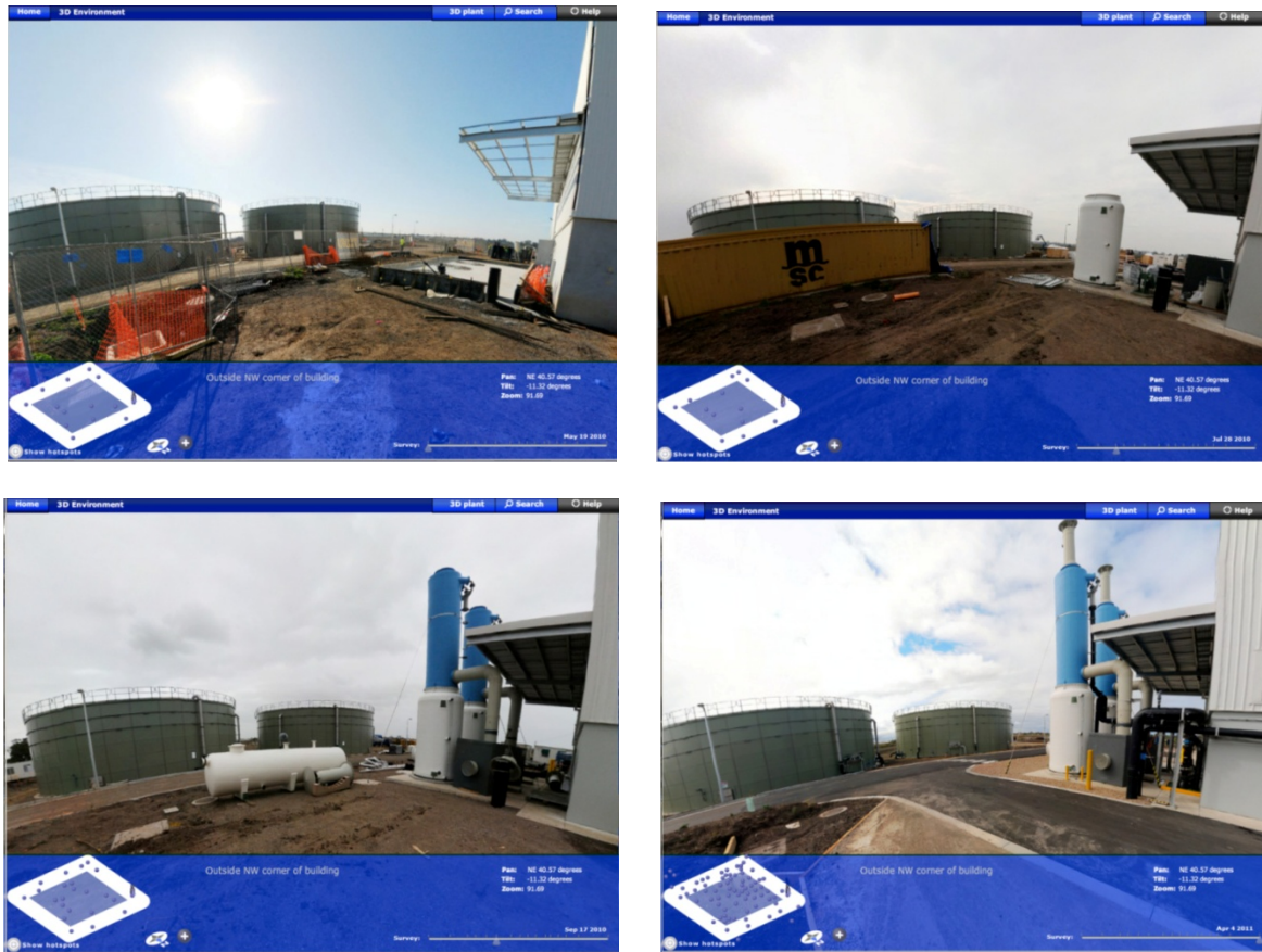
Figure 2. 4D time sequence of the installation of degasification towers in the City West Water environment, starting in May 2010 (top left) and finishing in April 2011 (bottom right).
