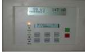
Figure 11. The control panel
